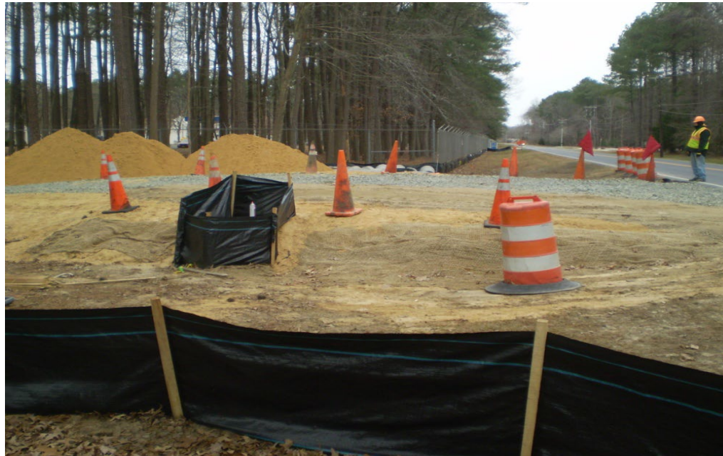
Silt fence installed at construction sites prevents storm water debris from entering local waterways and impacting surface water.
