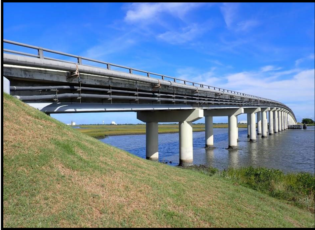
Photo 1-2. Photo of the Existing Causeway Bridge from the Southwest End of the Bridge Looking East.
