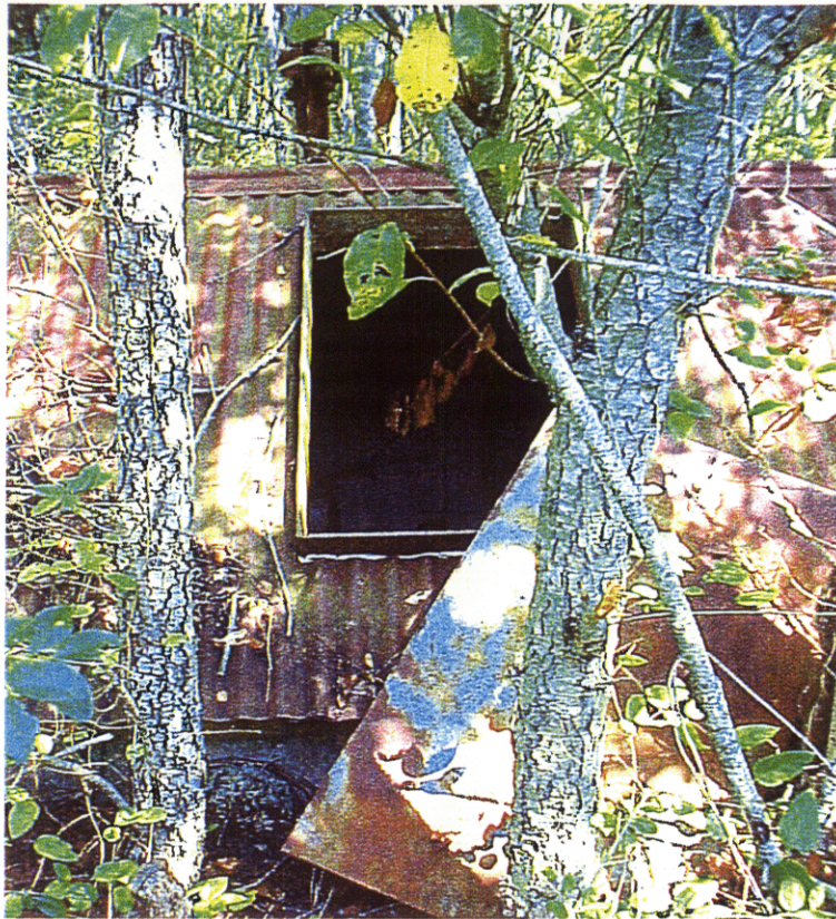
Figure 5.2-2. Site 3 – Two 600,000-Gallon Fuel Tanks – Site Conditions Photograph Wallops Flight Facility, Accomack County, Virginia
