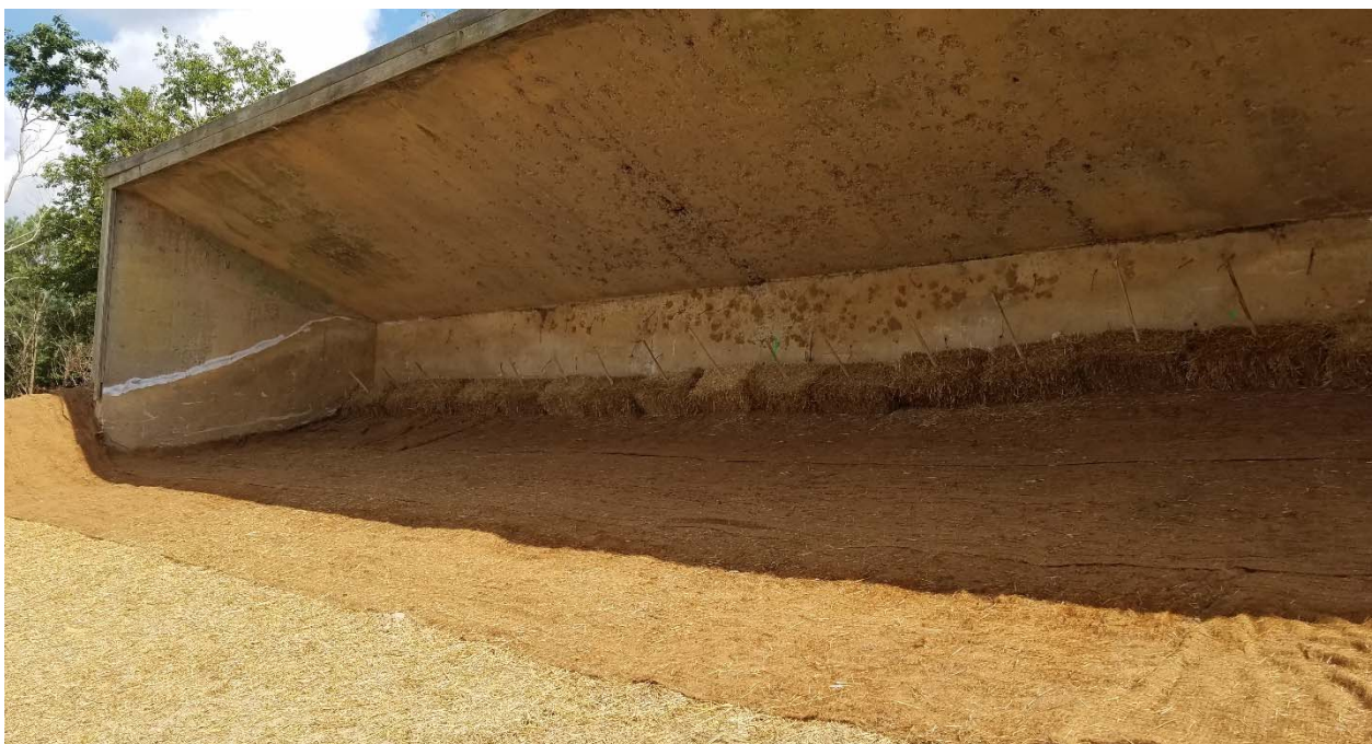
Photograph 26: Looking northwest at the target mound and concrete backstop at the Pistol Range. Hay bales were staked in to prevent erosion, as well as to keep the coconut fiber matting in place.
