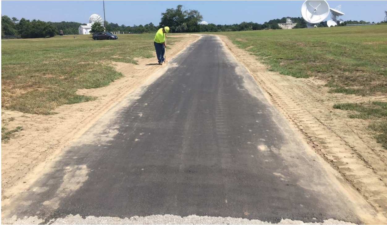
Photograph 56: Looking northeast down the asphalt road after the paving and site restoration was complete.
