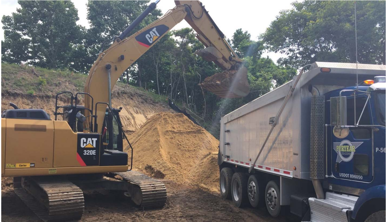
Photograph 36: View of lead-impacted soil being loaded into trucks for disposal offsite. It should be noted that the soil pile shown in the picture is clean backfill.
