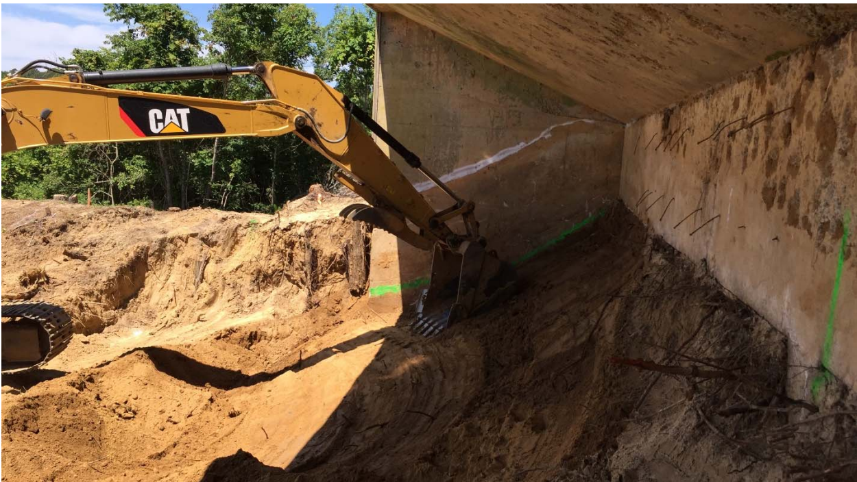
Photograph 14: Looking west at the Pistol Range target mound during the second phase of excavating in grid F3. The confirmation sampling revealed an additional 2 feet needed to be taken out. The green line on the concrete indicates the level of the soil after the first phase of excavating was completed.
