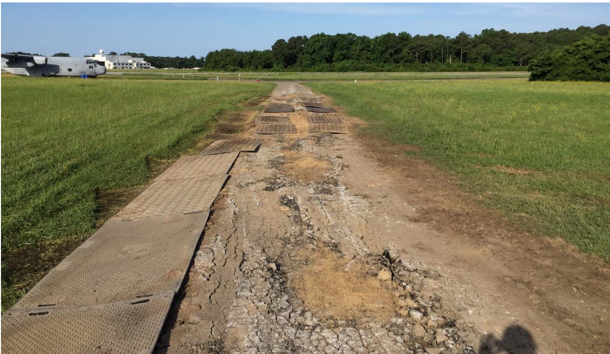
Photograph 49: Looking southwest down the asphalt road. Truck traffic deteriorated the road because no subbase was present.
