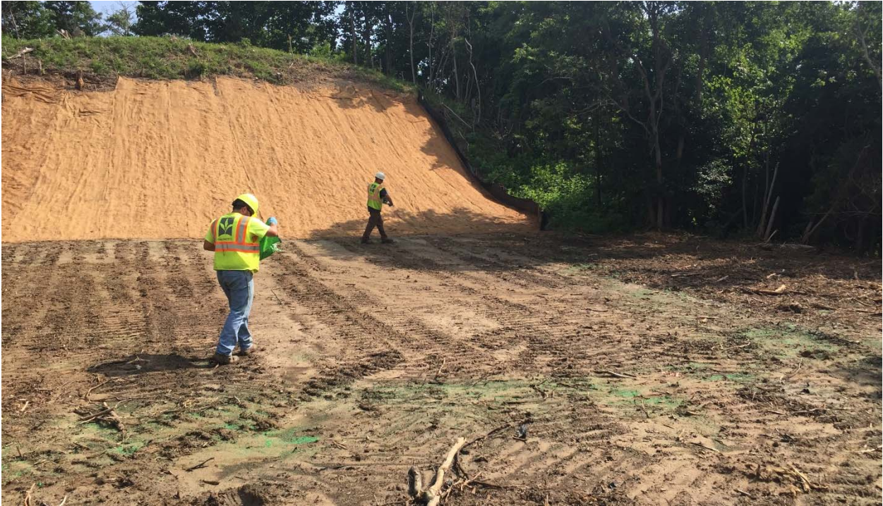
Photograph 42: Looking northeast at the Rifle Range target mound after it was seeded, fertilized, and coconut fiber matting was installed. In this photograph the flat portions are being seeded.
