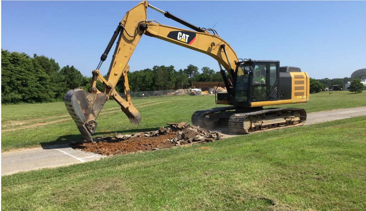
Photograph 50: Looking northwest as the excavator starts removing the asphalt from the damaged portion of the asphalt road. The asphalt was stockpiled onsite and eventually dropped off at a recycling facility.
