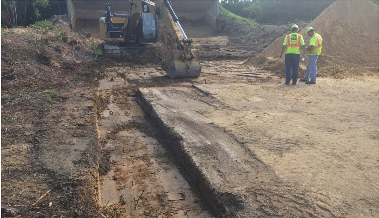
Photograph 17: Looking northeast at the excavated A3 and B3 grids at the Pistol Range with the stockpiled backfill on the right and the target mound in the background.
