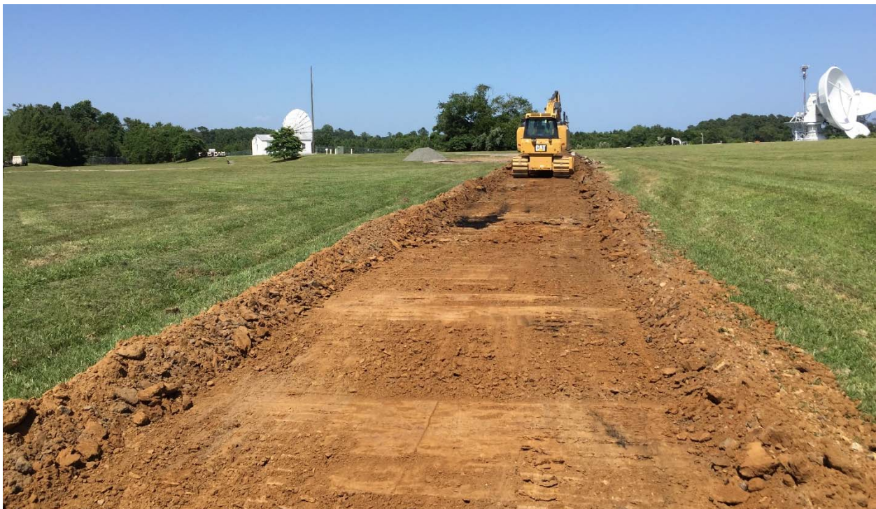
Photograph 51: Looking northeast as the bulldozer grades the damaged portion of the asphalt road.
