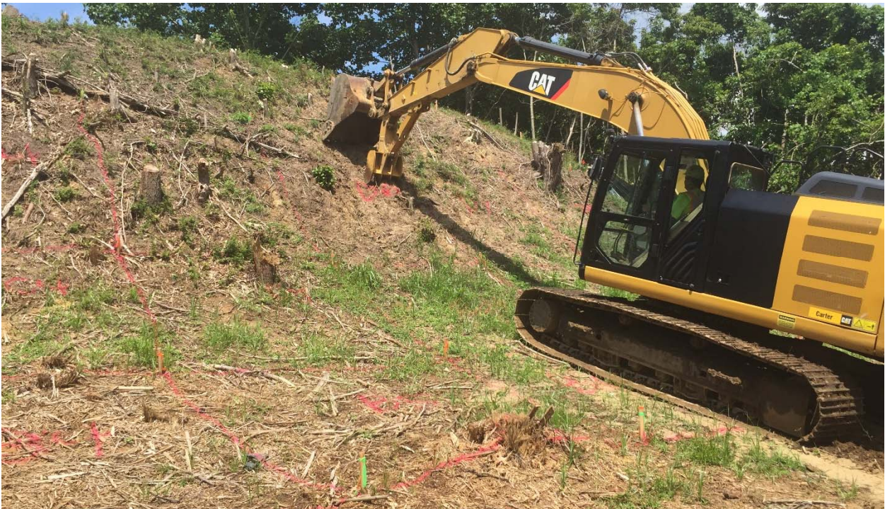
Photograph 33: Looking northeast at the Rifle Range target mound at the start of excavating. In this photograph the excavator is shown digging out grid D6.
