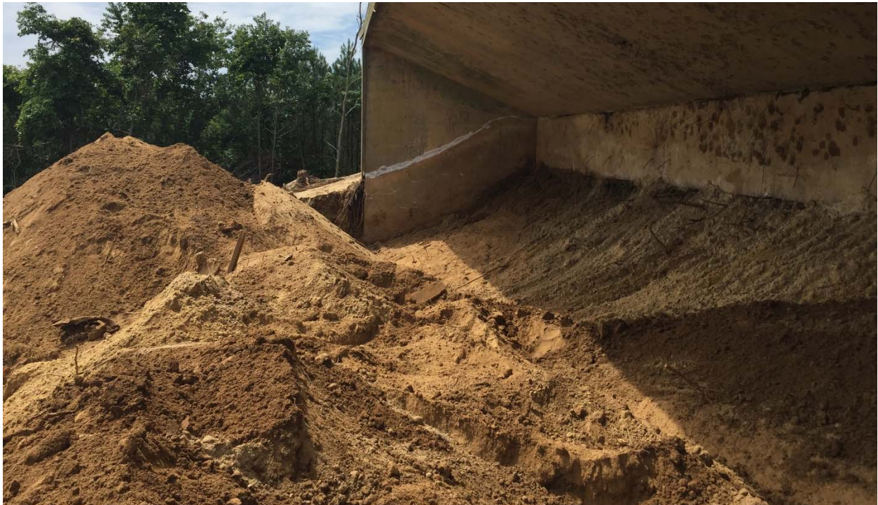
Photograph 10: Looking west at the Pistol Range target mound after the initial phase of excavating was completed at grids F2, F3, and F4. The white line on the concrete indicates the original grade of the soil.
