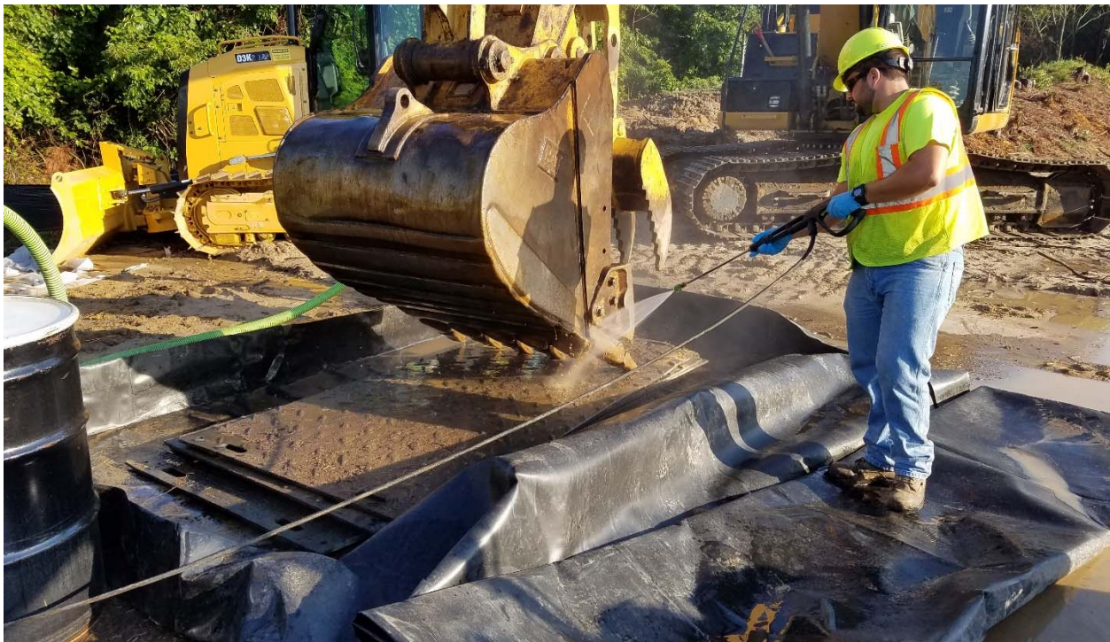
Photograph 18: Decontaminating the excavator bucket at the concrete pad after excavation activities were completed at the Pistol Range.
