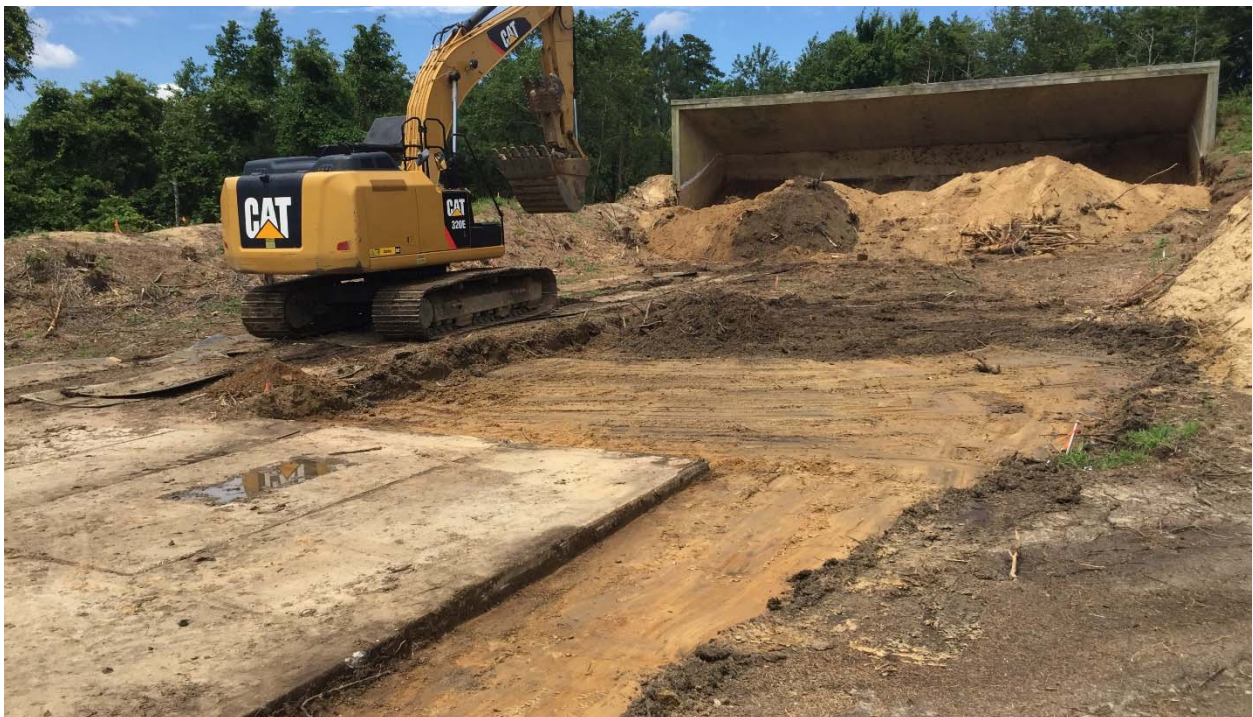
Photograph 16: Looking north at the excavated A4 and B4 grids at the Pistol Range. The stockpiled lead-impacted soils, target mound, and concrete backstop are visible in the background.
