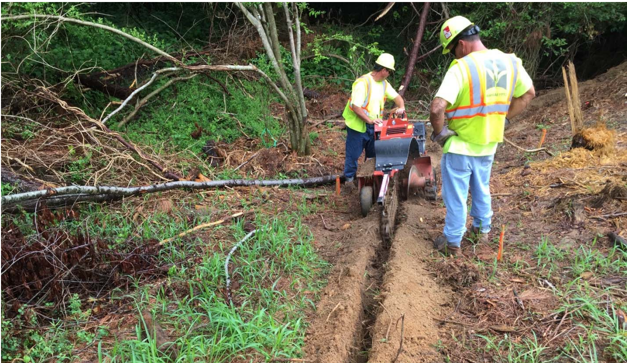
Photograph 31: Looking northwest at trenching activities in preparation for silt fence installation at the Rifle Range. The trench cut through the grid A1.
