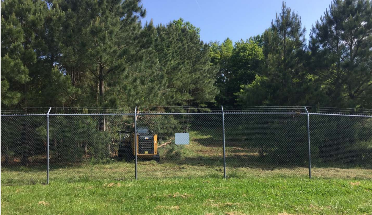
Photograph 28: Looking north at the Rifle Range at the beginning of tree clearing. The target mound is present in the background but is mostly concealed by the trees.
