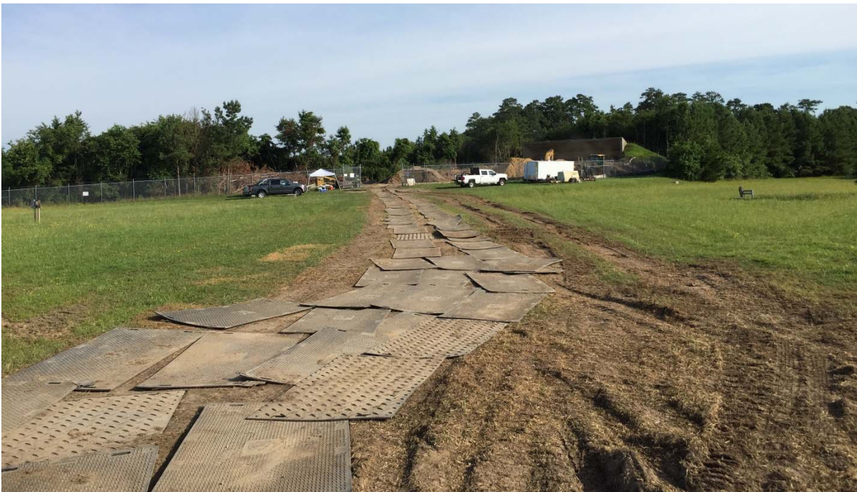
Photograph 45: Standing on the asphalt road looking northwest at the access road towards the gate to the Pistol Range. Despite the use of the traction mats the access road got rutted.
