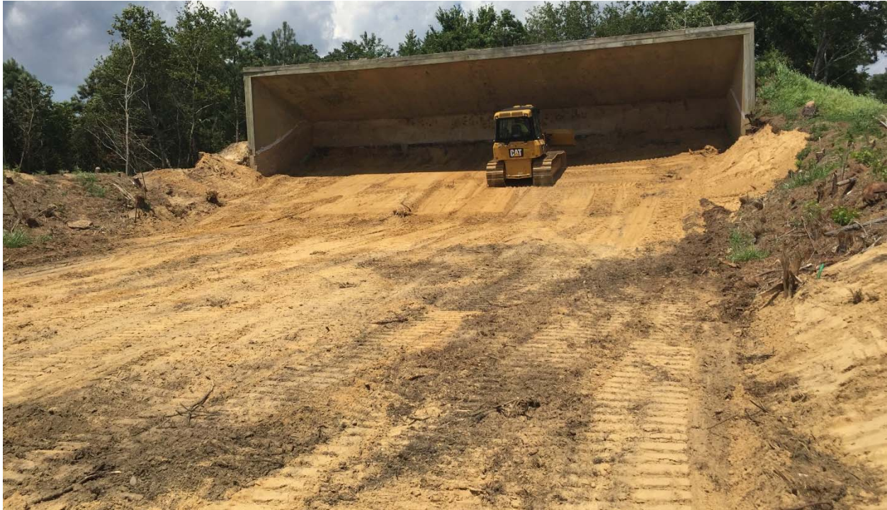
Photograph 21: Looking north at the target mound at the Pistol Range as the remaining backfill was spread and graded.
