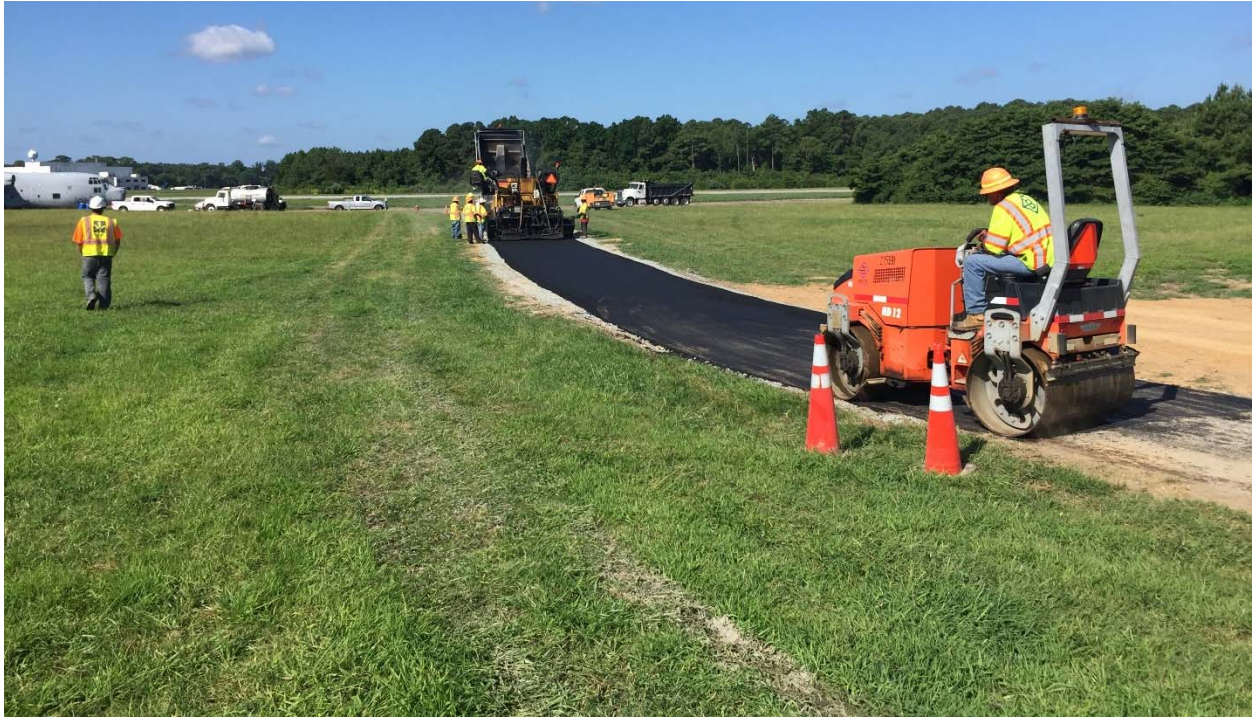
Photograph 54: Looking southwest down damaged portion of the asphalt road during the re-paving.
