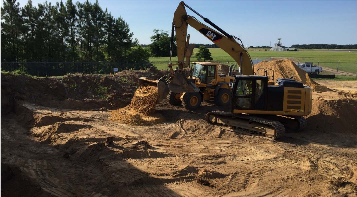
Photograph 13: Looking southeast during the backfilling of grids E3 and E4 at the Pistol Range. Confirmation samples were pending at grids F3 and F4 so backfilling was not started in these grids.
