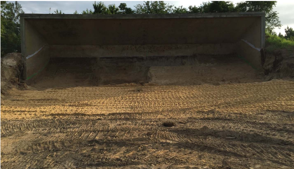
Photograph 20: Looking northeast at the target mound, concrete backstop, and the backfilled E3 and E4 grids at the Pistol Range.
