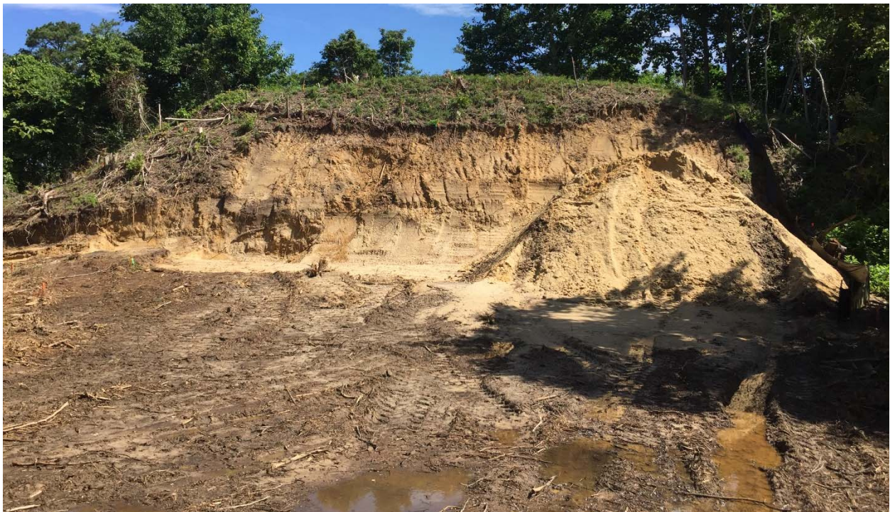
Photograph 37: Looking north at the Rifle Range target mound after all lead-impacted was hauled offsite. The soil stockpiled in the photograph is clean backfill.
