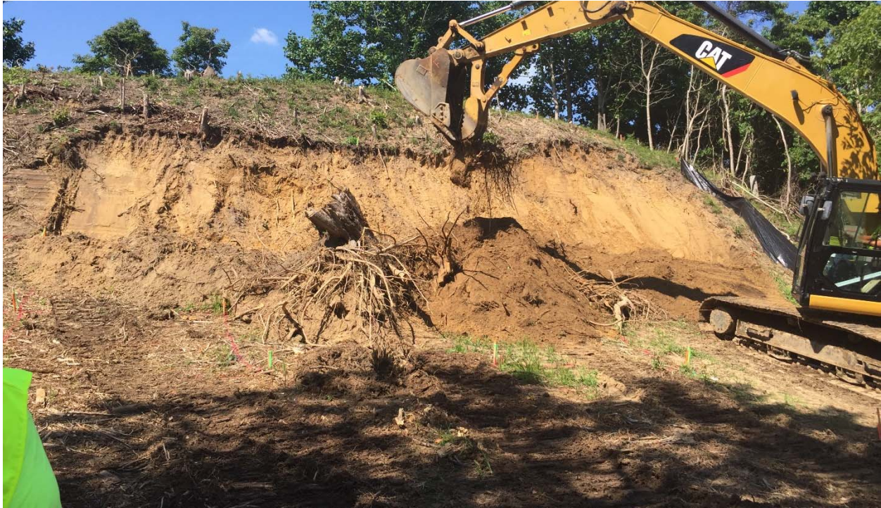
Photograph 34: Looking northeast at the Rifle Range target mound after grids D4 through D8 were dug out. The lead-impacted soil was stockpiled in grids B5 and B6.
