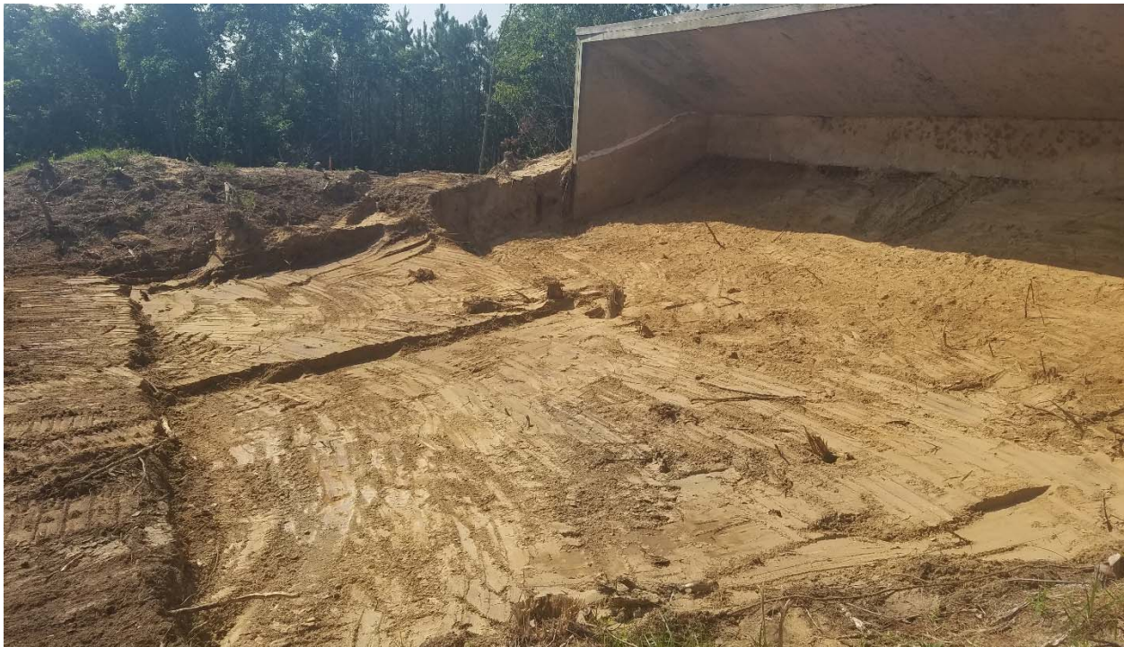
Photograph 12: Looking northwest at the initial excavation at the Pistol Range. This photo does not show the deeper excavation which took place later in grid F3.
