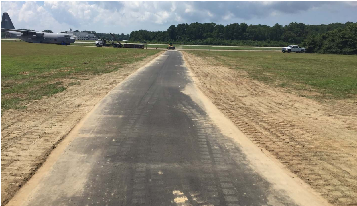
Photograph 55: Looking southwest down the asphalt road after the paving and site restoration was complete.
