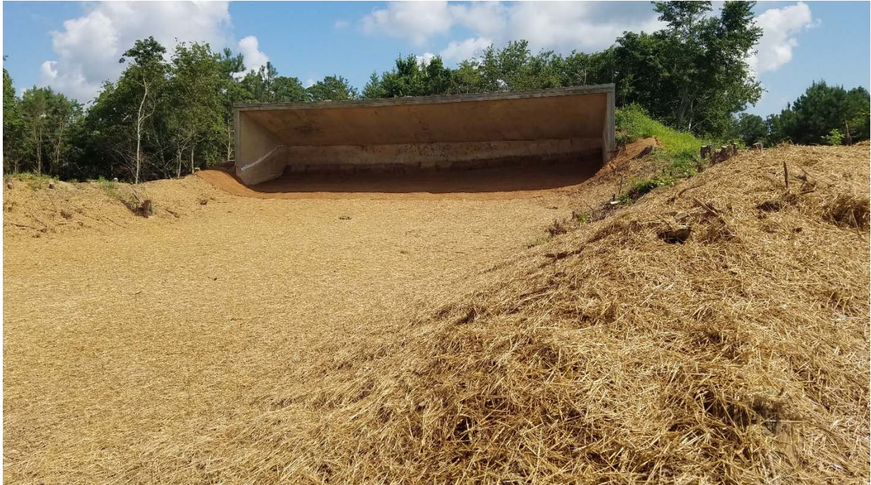
Photograph 25: Looking northeast at the target mound, concrete backstop, and berms after straw was spread and coconut fiber matting was installed at the backstop at the Pistol Range.
