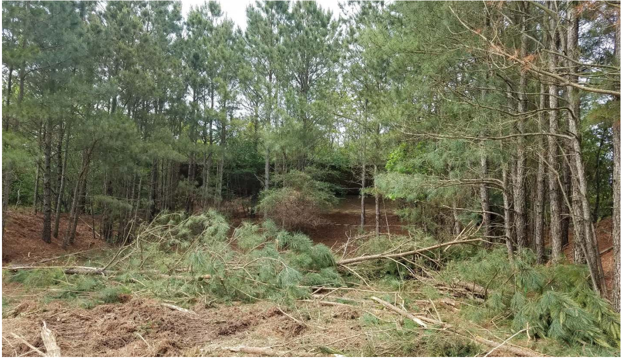
Photograph 3: Looking north at the Pistol Range target mound during tree clearing activities.
