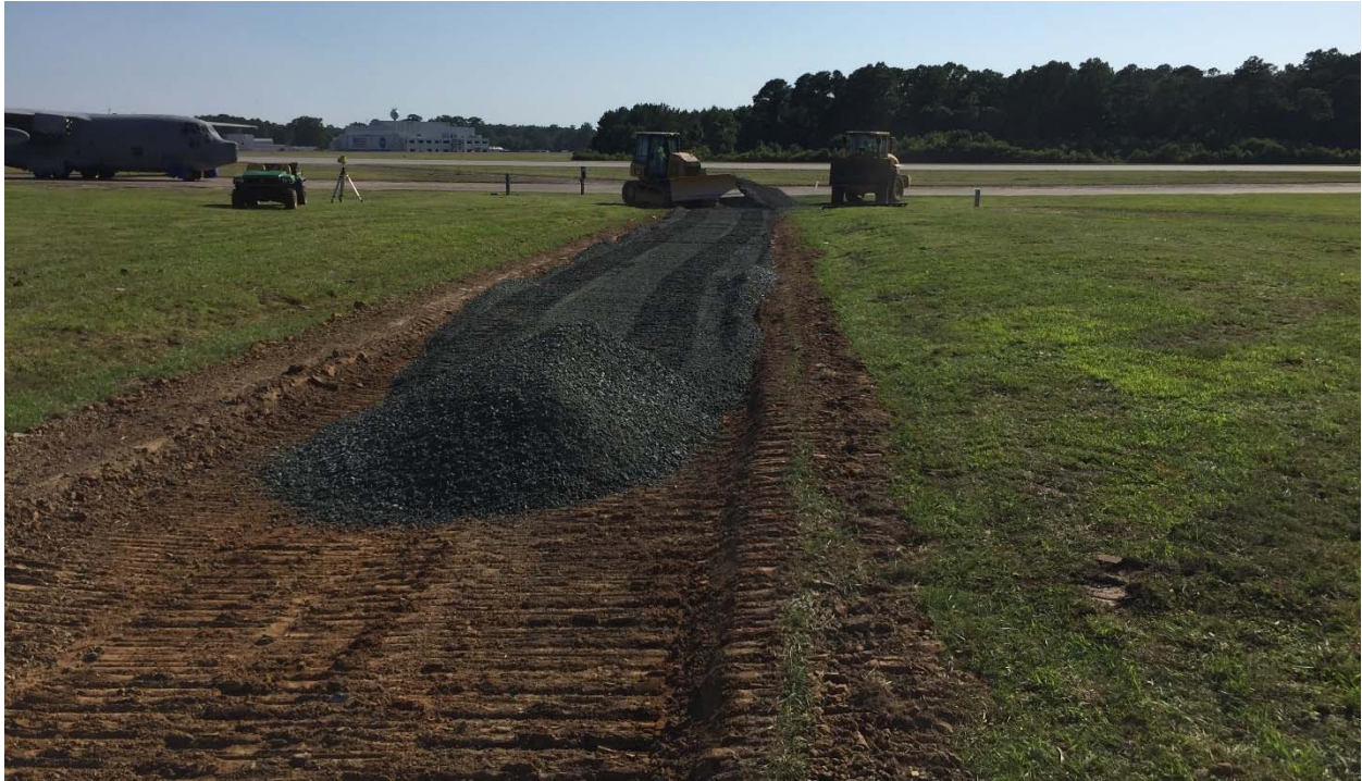
Photograph 52: Looking southwest as the bulldozer adds the subbase to the damaged portion of the asphalt road.
