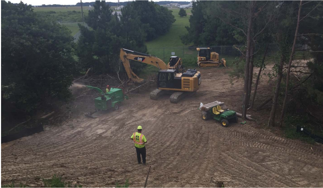
Photograph 40: Standing on the Rifle Range target mound looking south. The top soil has been spread and final grading was completed. In this photograph chipping of the stockpiled trees is being carried out.
