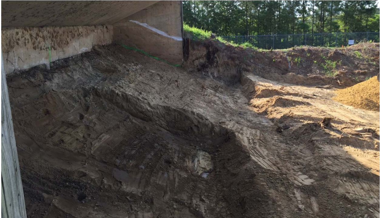
Photograph 15: Looking east across the target mound at the Pistol Range after grid F3 was excavated an additional 2 feet.
