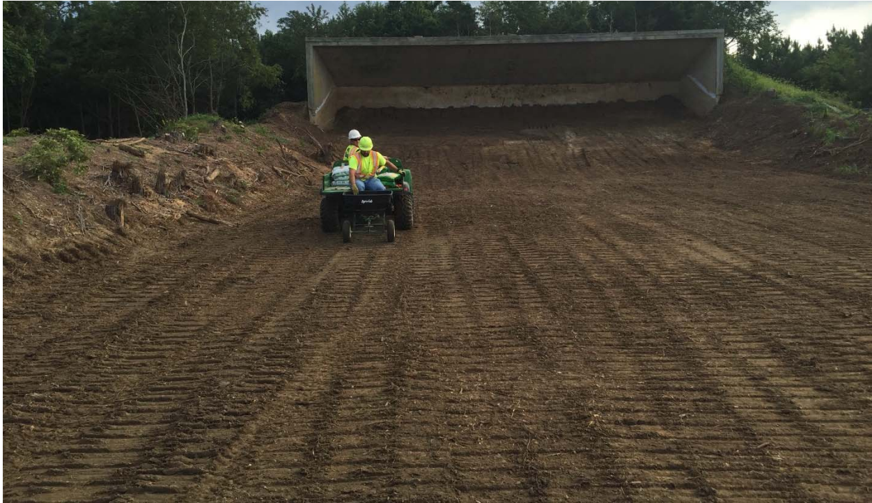
Photograph 23: Looking northeast at the target mound and concrete backstop during seeding after the top soil was graded at the Pistol Range.
