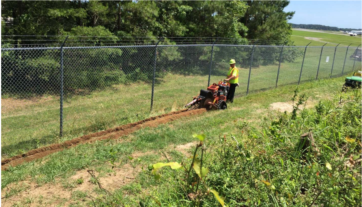
Photograph 5: Standing on the northern berm of the Pistol Range looking southeast at trenching activities in preparation for silt fence installation.
