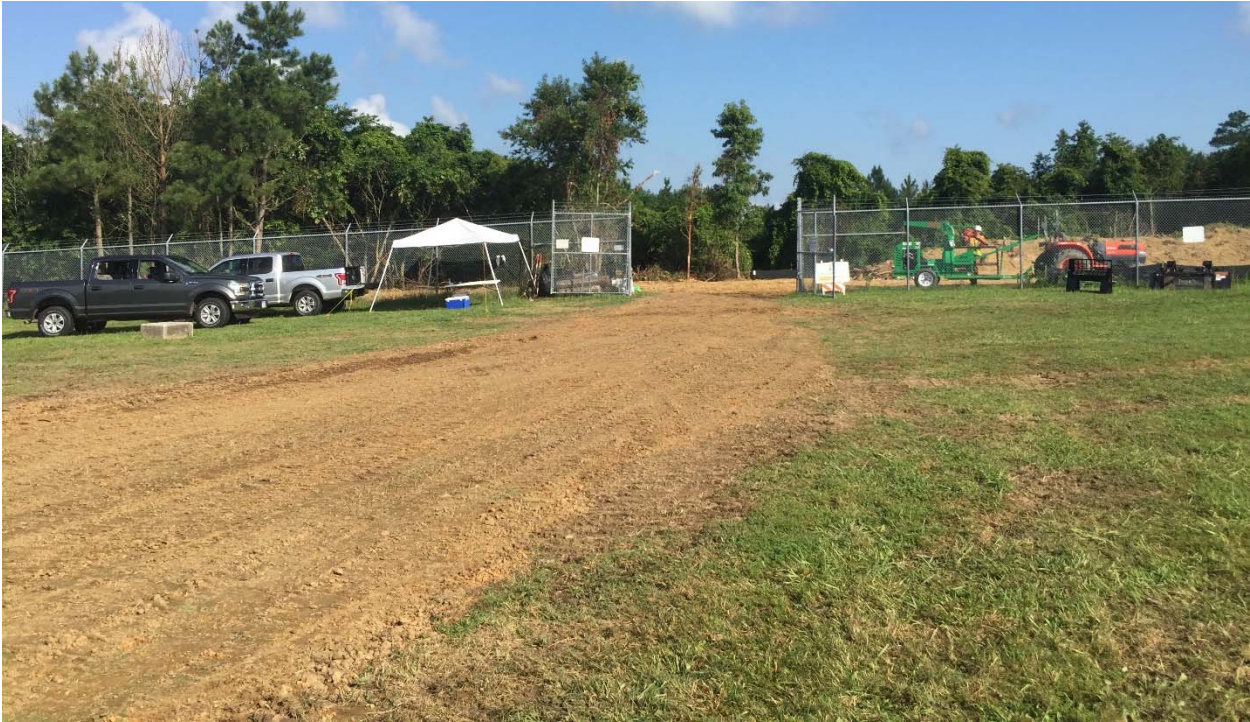
Photograph 48: View of the access road after restoration activities were completed. The disturbed areas were seeded and fertilized but no straw was spread due to concerns with airfield.
