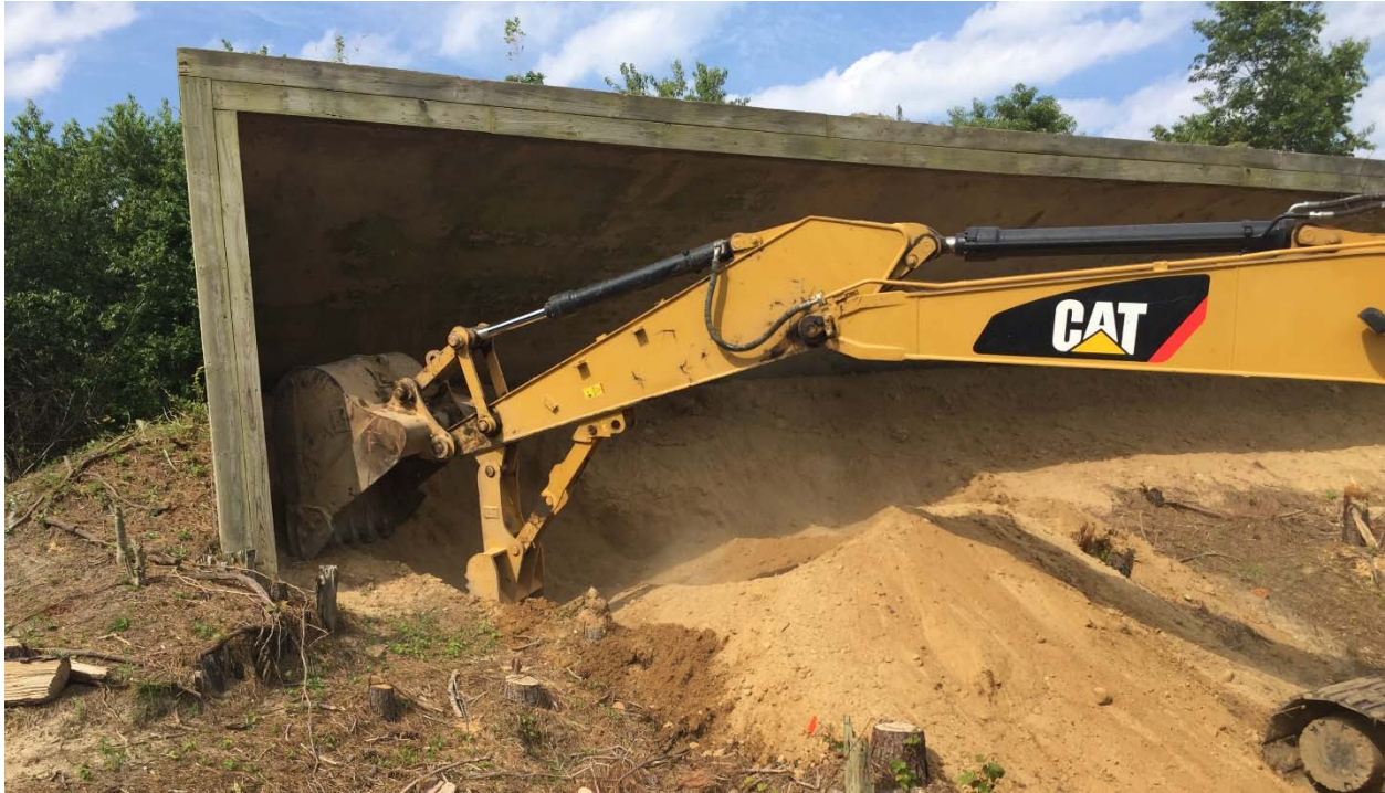
Photograph 9: Standing on the southern berm of the Pistol Range looking at the target mound during excavation of grids F2 and F3.
