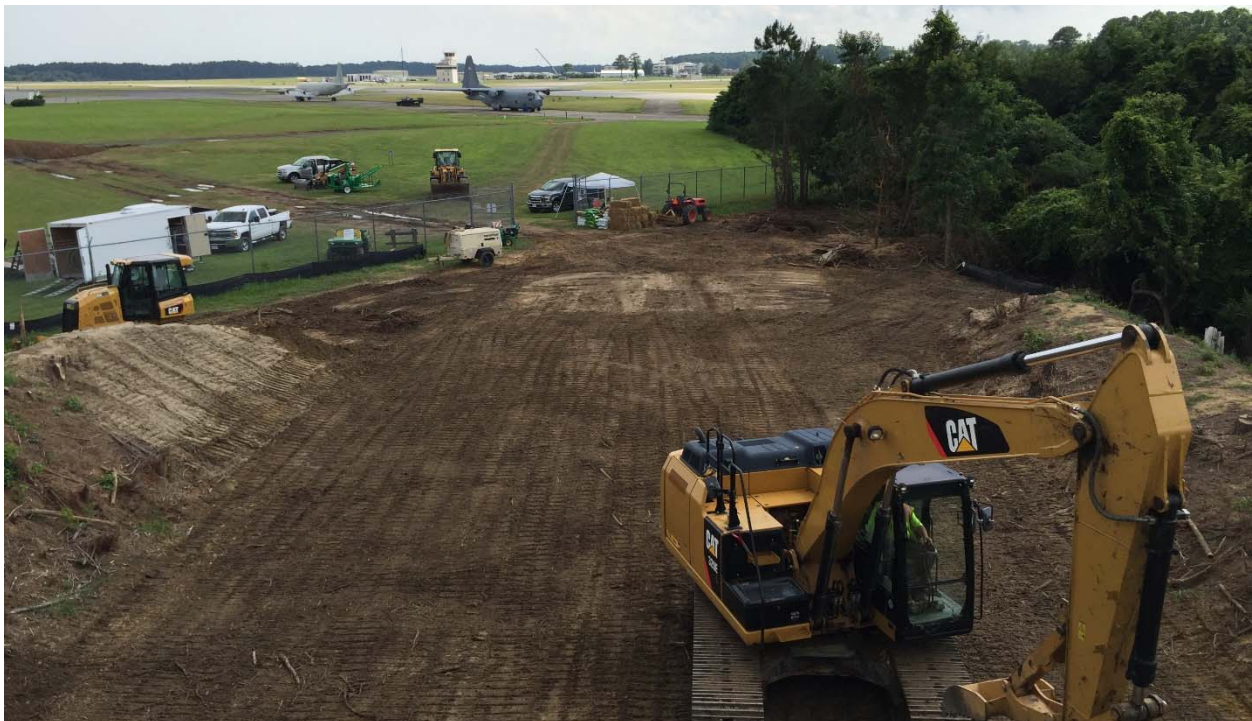
Photograph 22: Standing on the concrete backstop looking southwest across the Pistol Range. The top soil was spread and graded. The access roads and support area can be seen in the background.
