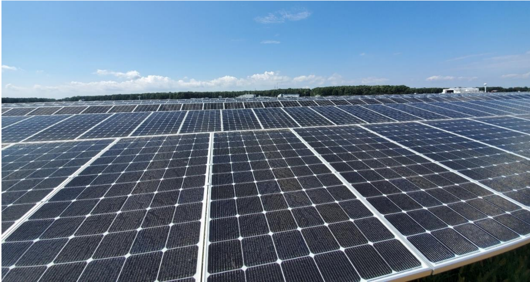
Wallops Airfield Phase 3a Photo Voltaic Panels
