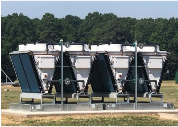
WFF E Buildings Dry Cooler
