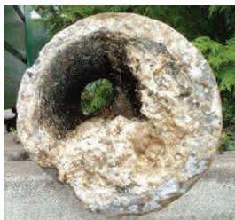
FOG Clogged Pipe
